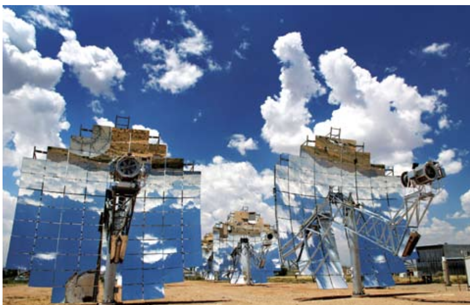
Parabolic trough for concentrating solar power
